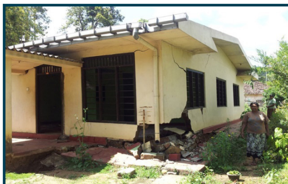
A DISTORTED HOUSE AS PER THE UMA OYA FAILED PROJECT
